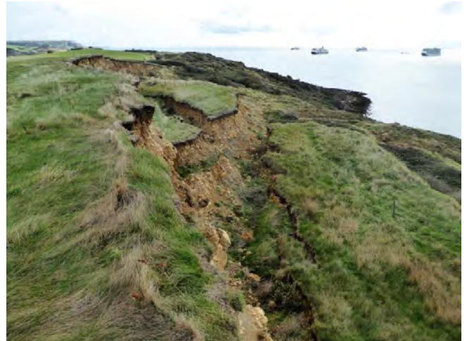
Land slippage east of Swanage, Credit: Alan Holiday
