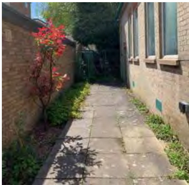
Uneven paving in the passageway, Credit Bruce Longstaff
